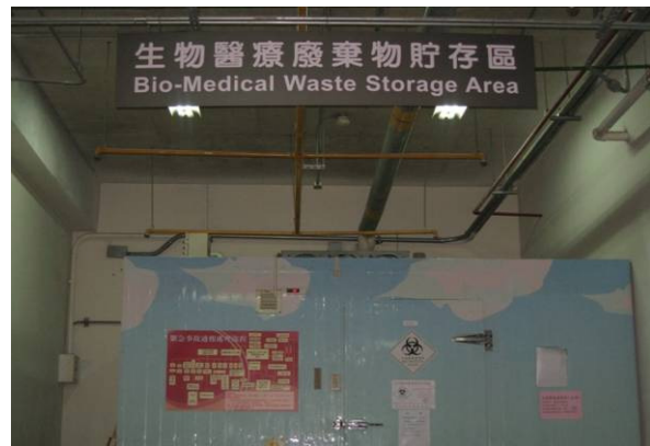
Shuang Ho Hospital- The general waste handling area and biomedical waste storage area.
