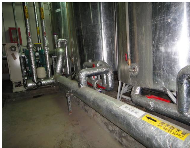
Mackay Memorial Hospital Tamsui Branch- Heat pump system
