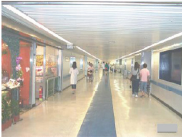
Chang-Gung Memorial Hospital- High efficiency, disaster- proof electrical lighting equipments
