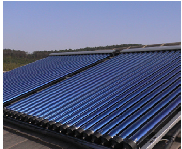
Alexandra Health Cluster- Solar thermal system
